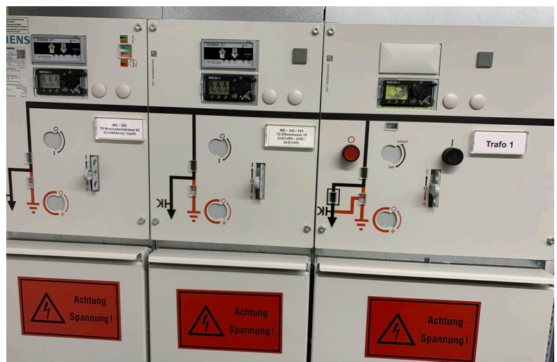
Brunnadernrain transformer station after renovation
