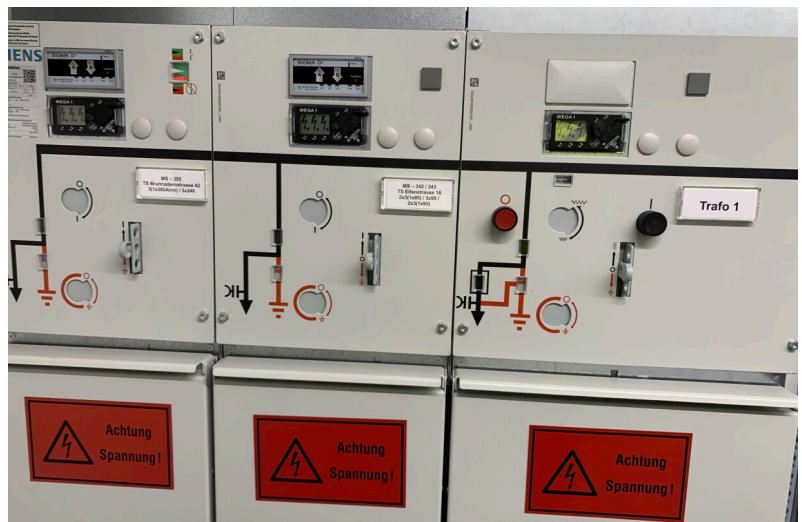
Brunnadernrain transformer station after renovation
