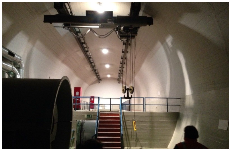
Centrale Aria Tunnel San Bernardino
