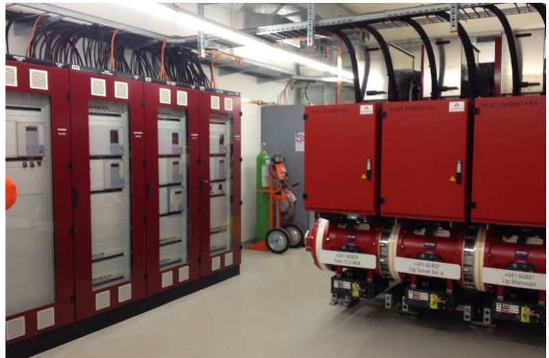
Locali Media Tensione Tunnel San Bernardino
